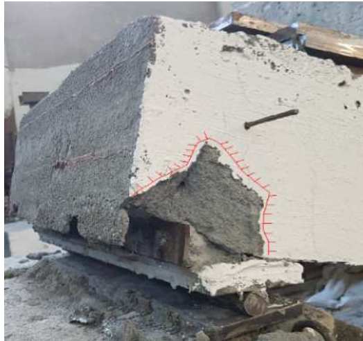
Figure 7. – A photo of concrete crumbling with anchorage corner around the support point
