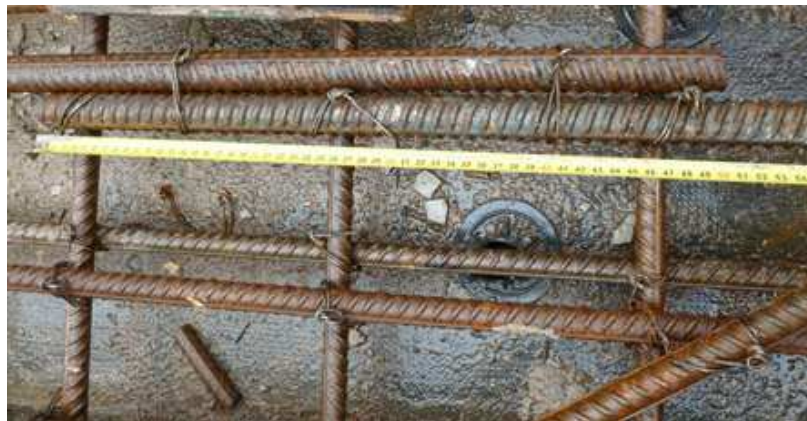
Fig. 1. Joints of valves without welding, The OVERLAP of rebar
